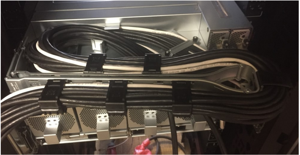
Figure 57. Cables routed through CMA baskets
